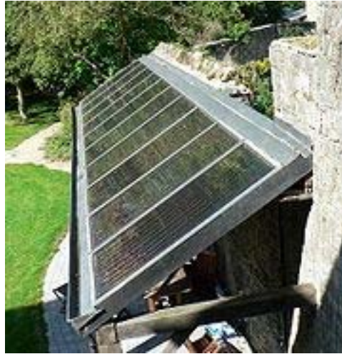
Solar water heaters
