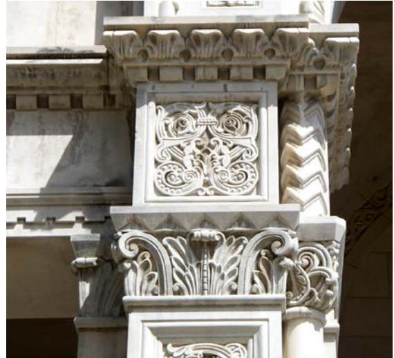
Figure 1L. Very elaborated decorative patterns, apparently of very classical or Rococo style, in the columns of many old buildings.
